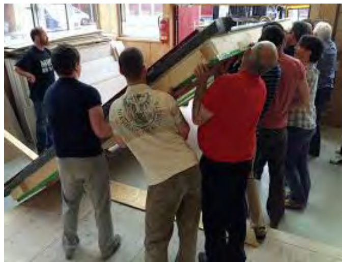
REMSOP F1 Group May 2014 Erecting a new retrofit panel for external cladding application
